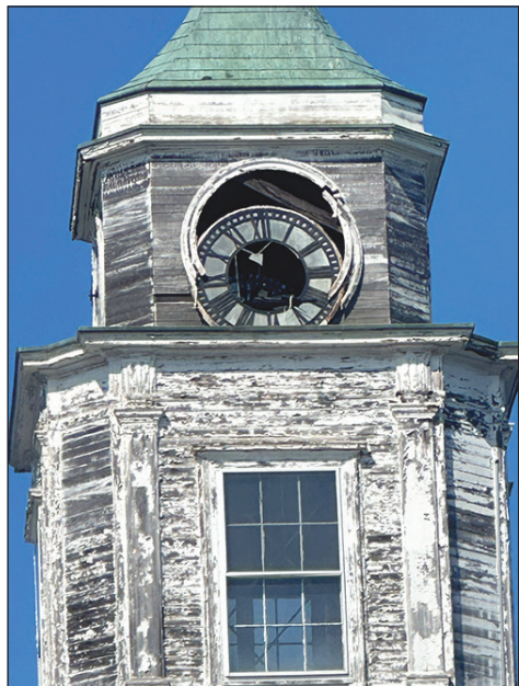
A windstorm last September caused damage to one of the clock faces.
